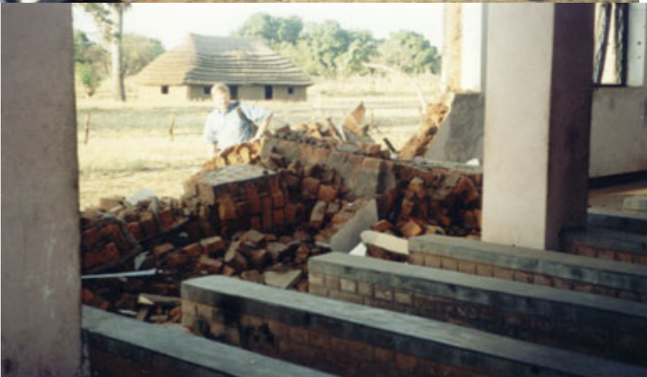
Fraser Cathedral Bombed by the South African Air Force on 16 June 1944. The building was severely damaged and the interior, including the altar, was destroyed.
